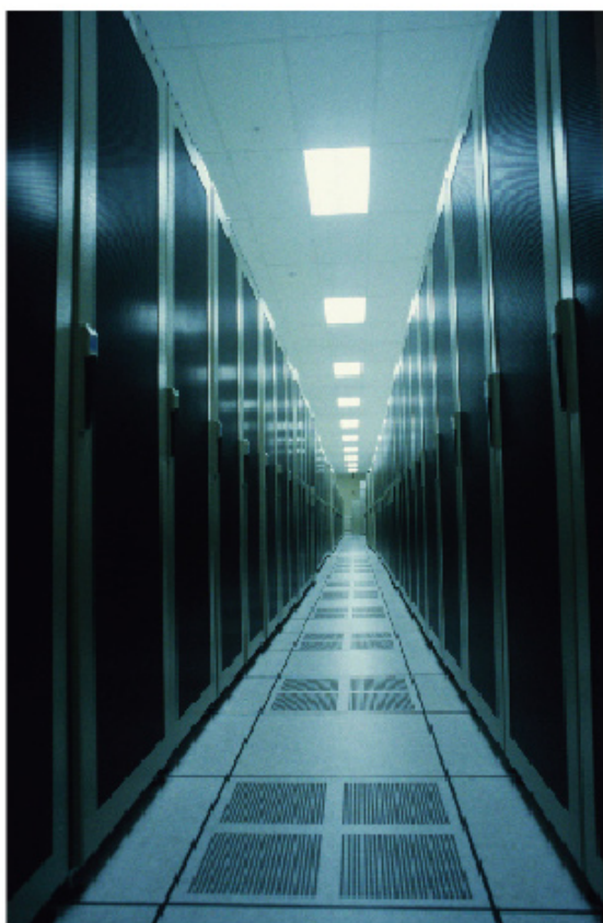
Typical data center—Half of its energy to run computers and the other half to cool them
